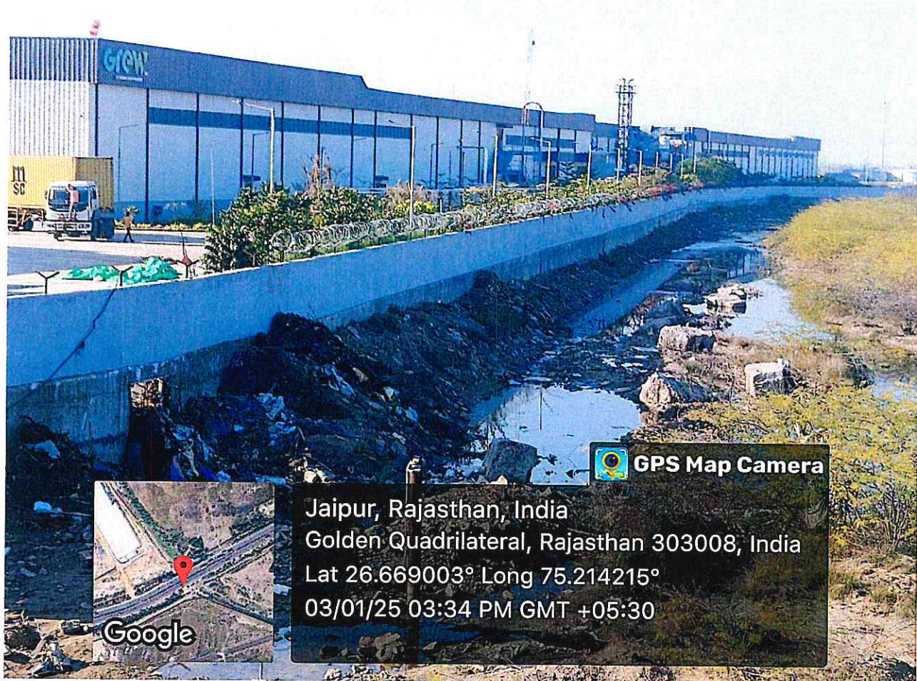
R-7 dumping waste openly leading serious threat to environment
